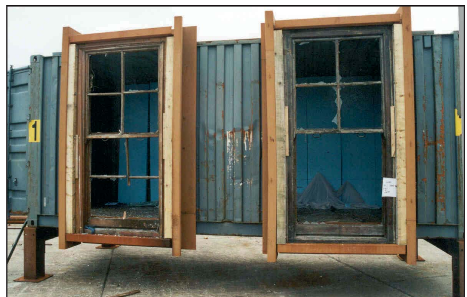
The effects of blast damage can be clearly seen on these windows at a UK explosives research facility.
